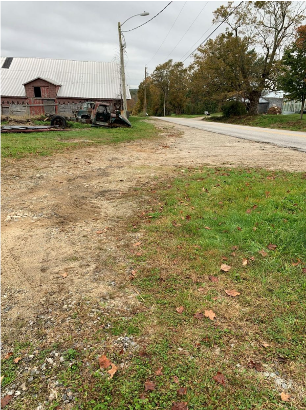
Overflow water washes out drive and heads back to edge of road.
