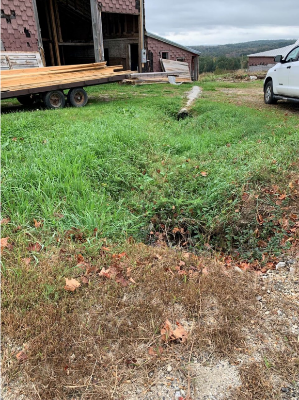
Town road culvert outlet heading to pipe added by previous owner.
