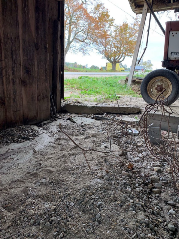
Water flows into lower barn main floor. Note deposited sediment
