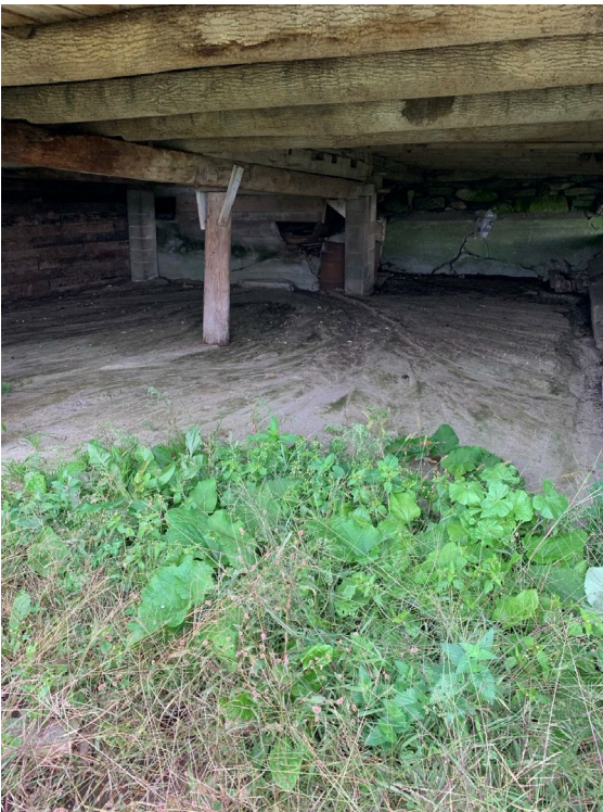
Basement of barn. Note fine sediment and rill lines.
