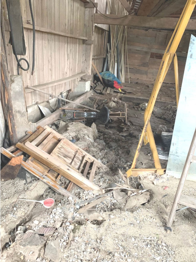
Note gully in sediment from rushing water into barn. Water drops down along wall and into open basement.
